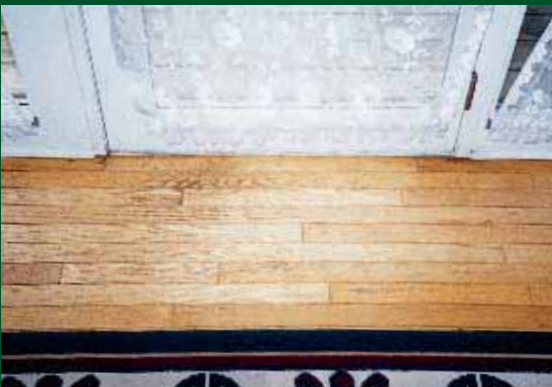
Dirty floors with finish totally worn off.
