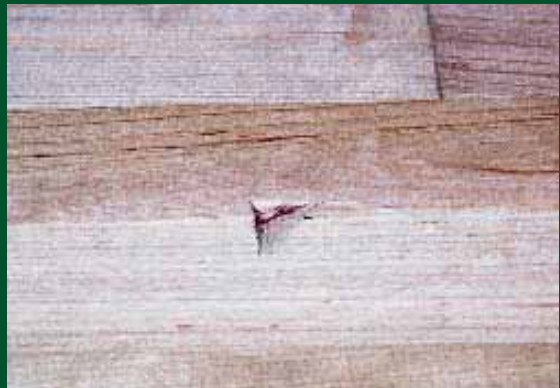
Dents (these usually require board replacement).
